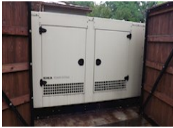
Kohler Power Systems generator
