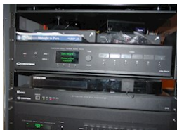
Crestron Cen-Track multi-tuner
